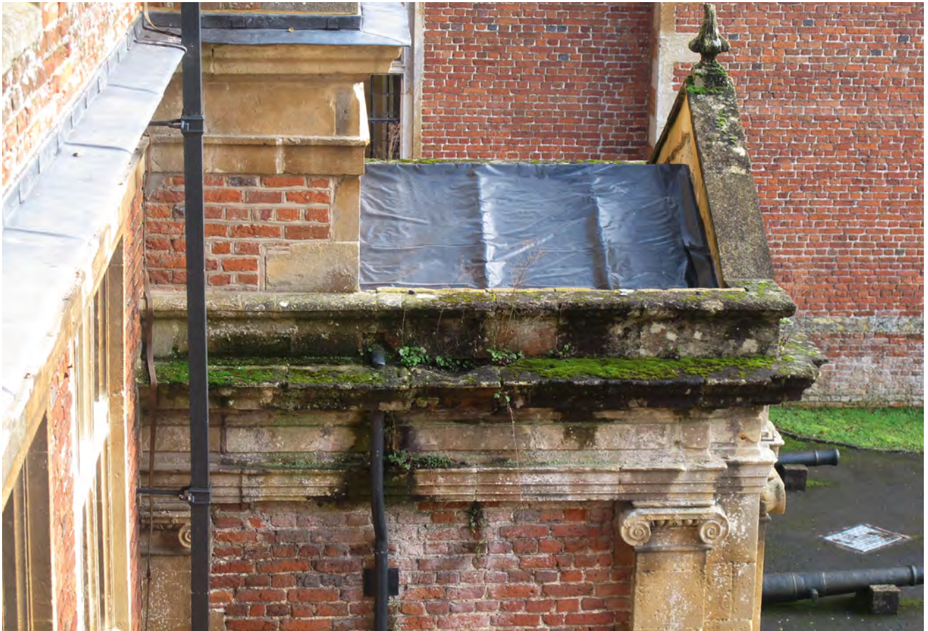
Figure 7: Poor maintenance (image © Historic England)
