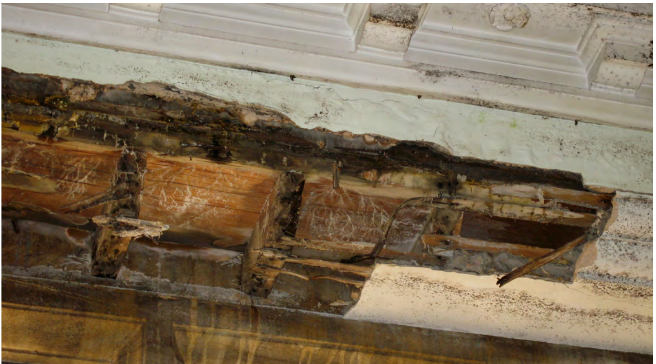
Figure 8: Collapsed plaster due to water penetration via lead parapet gutter (image © Historic England)
