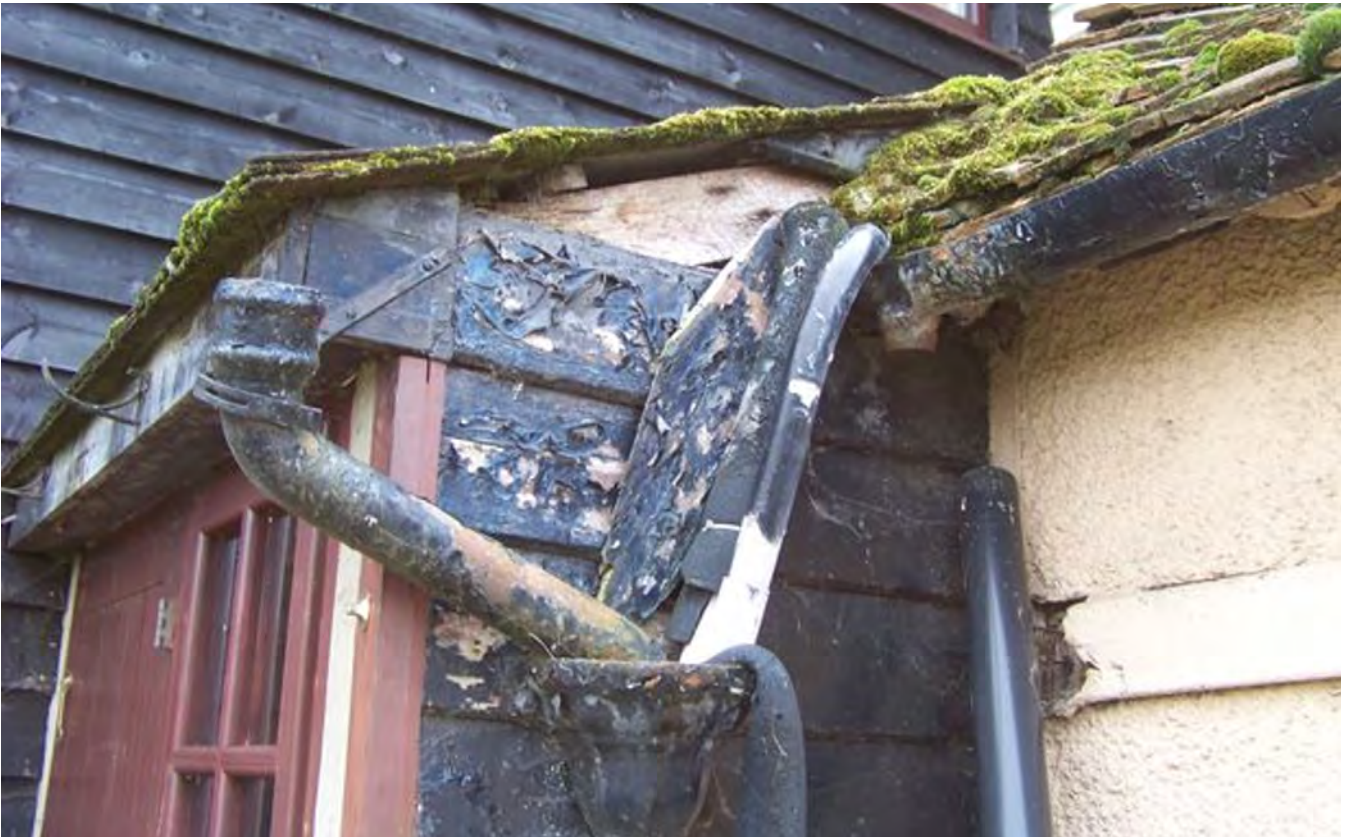
Figure 5: Defective rainwater gutters and downpipes (image © PCA)
