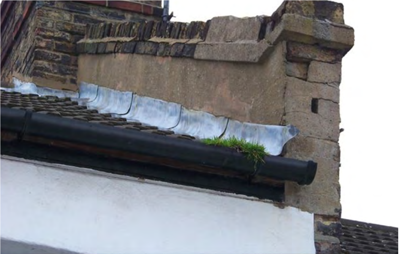
Figure 1: Parapet wall in poor condition (image © PCA)
